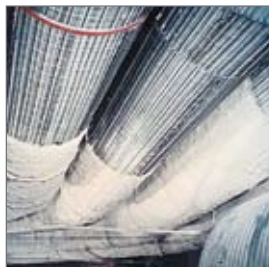
Protection incendie Fire protection
